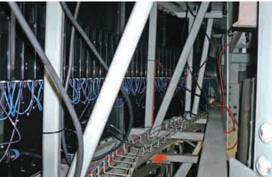
In a rare look from behind the LED facade, the individual LED modules, and their steel-frame modules, can be seen.
